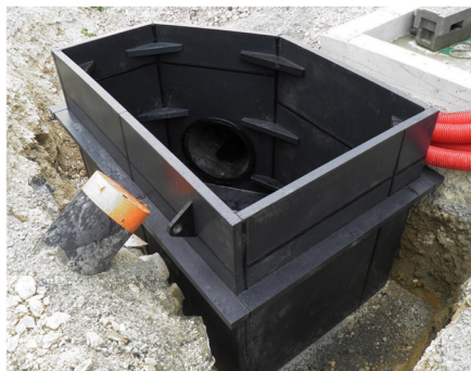
RAIN WATER TANK
